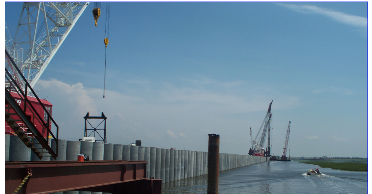
Concrete Cylinder Piles form the New Orleans IHNC Floodwall; Work Trestle in foreground. Photo courtesy of Foundation Testing and Consulting.
